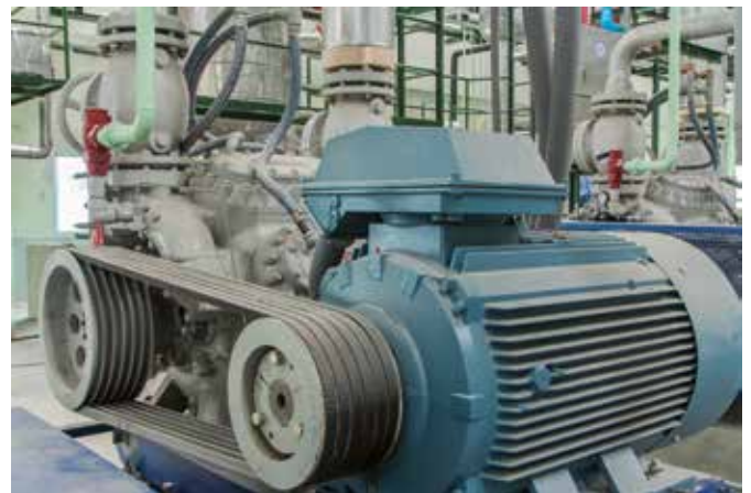
Industrial cooling system
